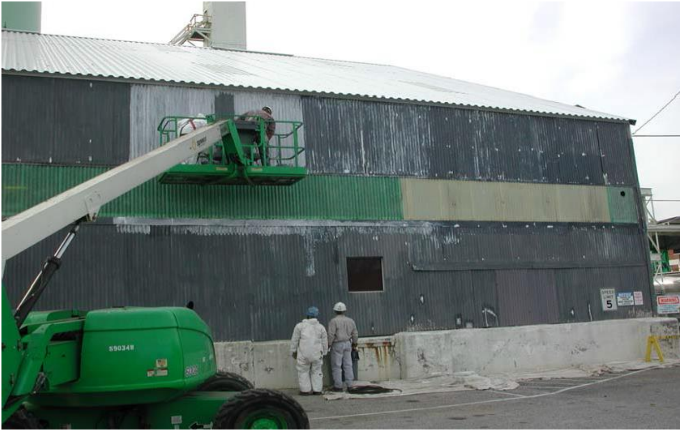
The F-50 Penetrating Stabilizer Primer was applied to all exterior surfaces, including all of the repaired areas.
